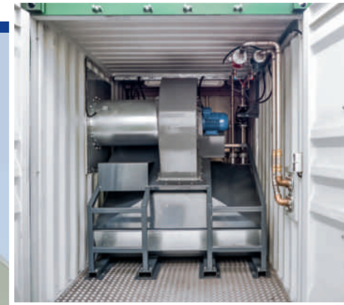
Supply air with heat exchanger and blower
